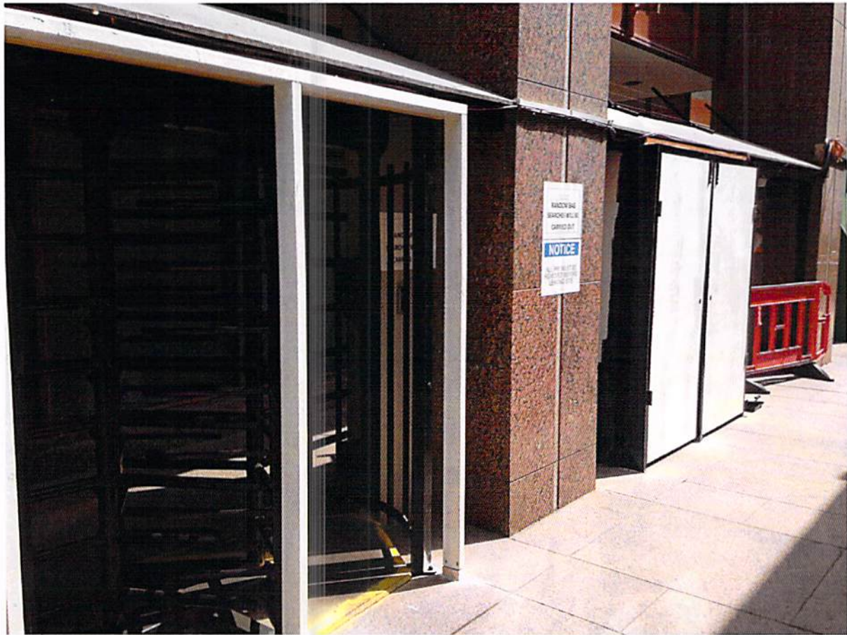
Photo 2 - Photo taken from inside the site showing a turnstile without the demountable panel installed and a turnstile with the demountable panel in place.
