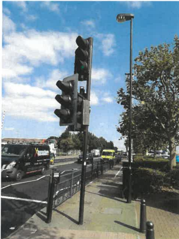
Unobstructed lamp column at the controlled crossing point.
